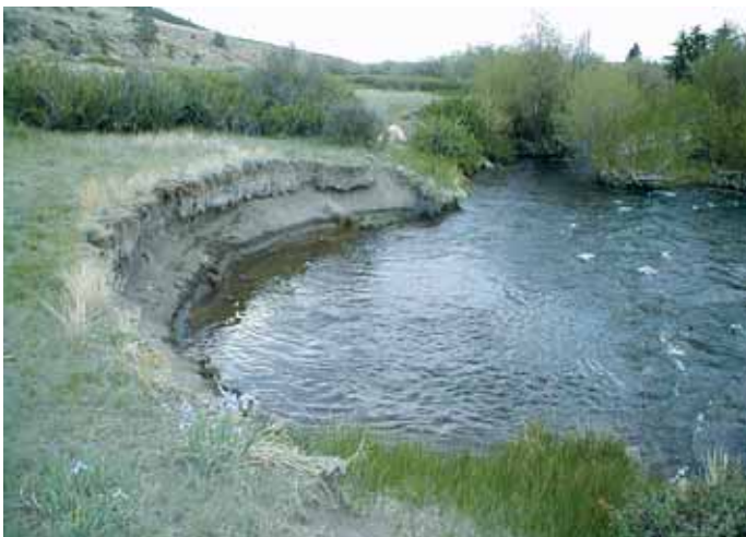
This streambank is severely eroded due to accelerated water velocity from newly installed upstream riprap.
