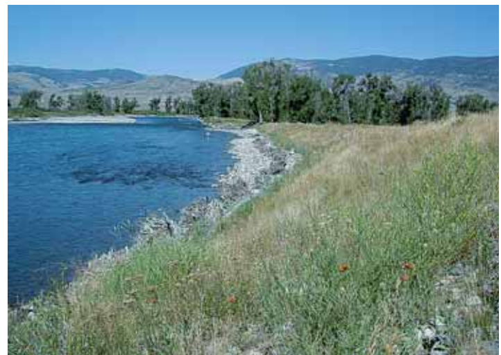
After: Turf reinforcement materials, an erosion-control blanket, wood material and native seed blends were used to restore the 1,200-foot streambank.
