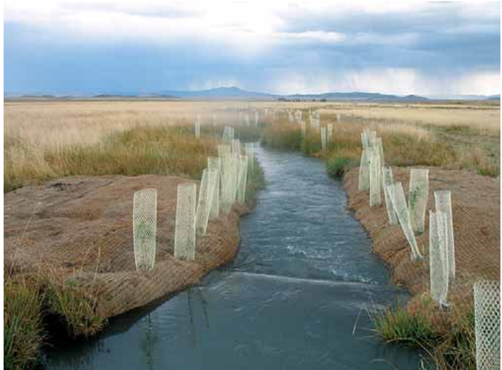
Erosion-control blankets and cottonwood saplings are used to stabilize this streambank. As the trees mature, the roots will help stabilize the banks and the trees will shade the stream, both cooling it and offering fish cover from predators.
