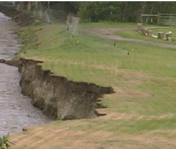
Severe riverbank erosion
